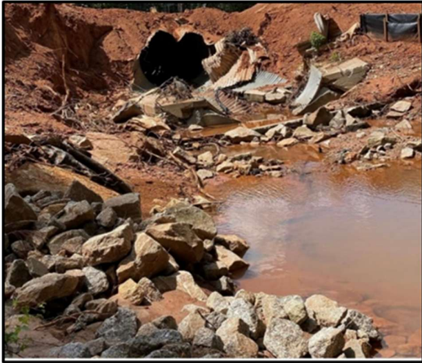
Partial Culvert Collapse 12 FOOT diameter
